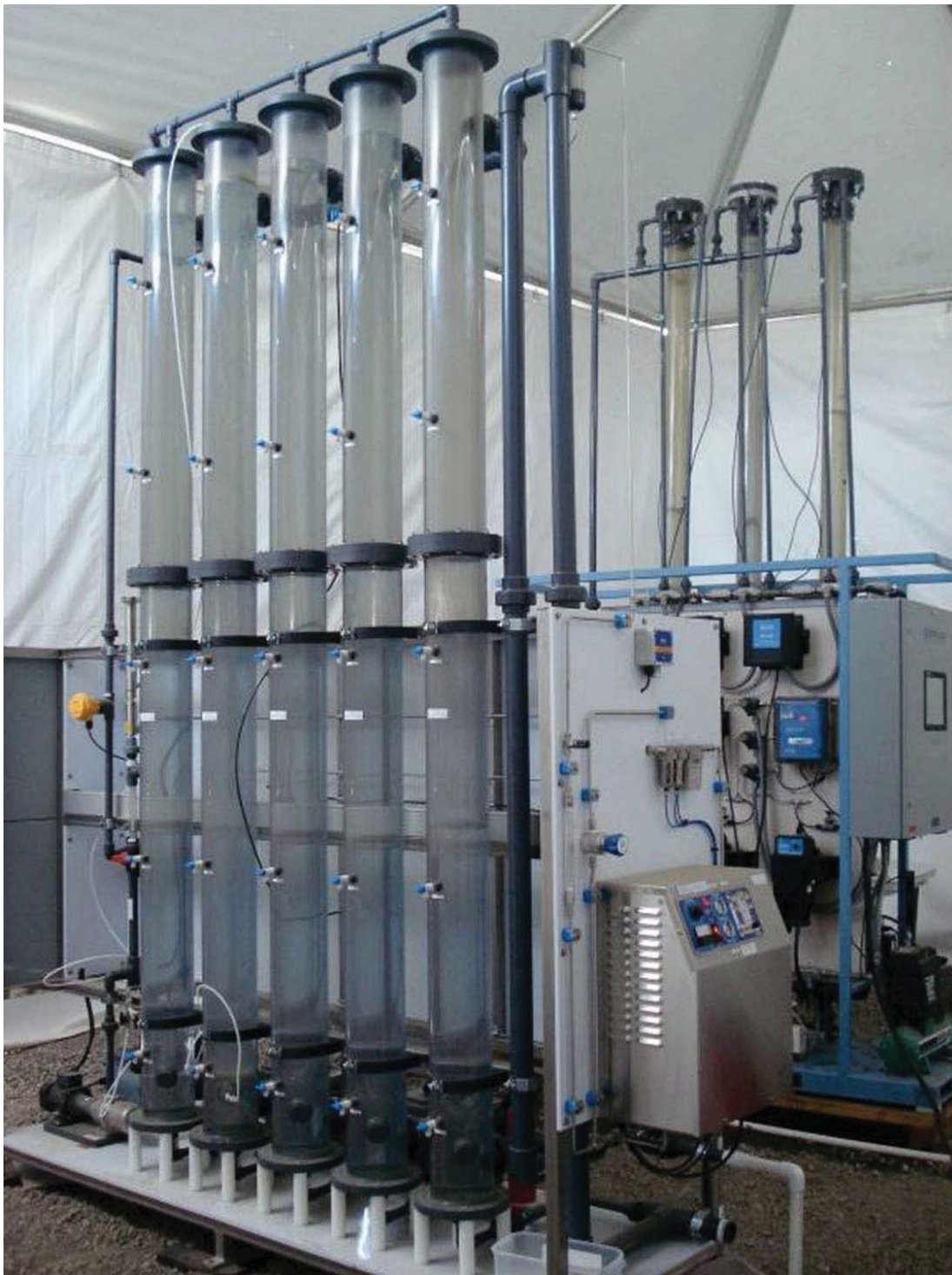
Figure 4 INTUITECH OZONE MODULE Z100 SET UP ON SITE AT BOLLMAN WTP CALIFORNIA DEPARTMENT OF WATER RESOURCES CALIFORNIA DEPARTMENT OF PUBLIC HEALTH
