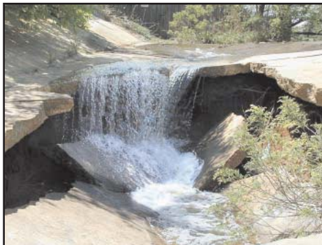
Knight Lake's crumbling spillway is indicative of numerous deficiencies in the west Oklahoma City dam.
