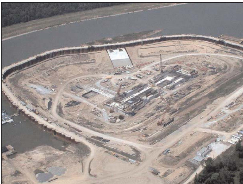
An aerial view of construction on Montgomery Point Lock and Dam. (Photo courtesy Arkansas Basin Development Association, Inc.)
