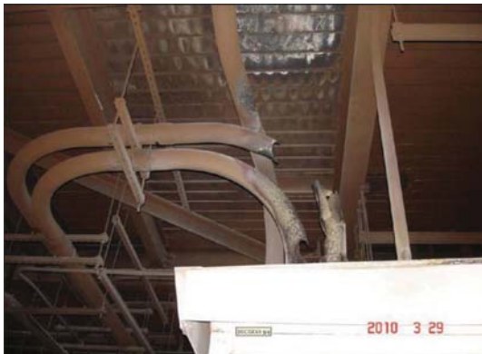
Conduit for electrical cables damaged by the fire at the HB Robinson plant. NRC photo.
