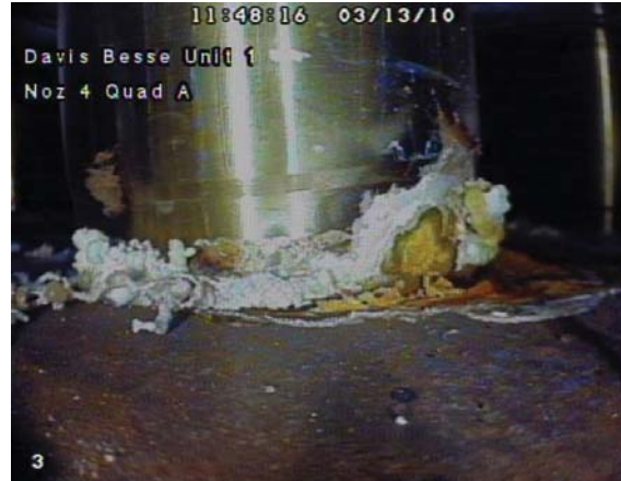
White-crystalline boric acid leaked through a cracked nozzle in the head of the reactor vessel at the Davis-Besse plant in Ohio. NRC photo.
