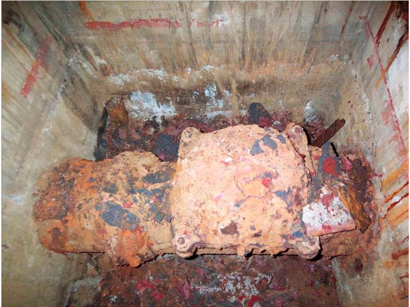
This July 2007 photo made available by the Nuclear Regulatory Commission in response to a public records request by The Associated Press shows a badly rusted valve inside a vault at the Indian Point 1 nuclear plant in New York state. The pipe was part of a containment spraying system that was initially a focus of concern as workers tried to find the source of leaks at the site. Leakage was eventually traced to spent fuel pools. The reactor had been shut down since 1974. (AP Photo/Nuclear Regulatory Commission)
