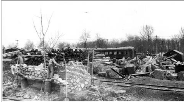
Keystone / Getty Images 1976: Workers start rebuilding work following earthquake damage in the Chinese city of Tangshan, 100 miles east of Pekin, with a wrecked train carriage behind them. (Photo by Keystone/Getty Images)
