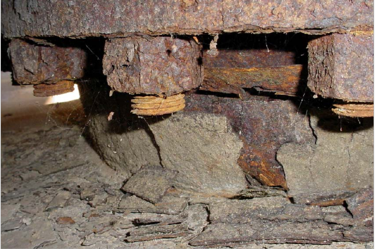
This June 14, 2007, photo made available by the Nuclear Regulatory Commission shows some of the extensive rust that accumulated on piping carrying essential service water at the Byron nuclear plant in Illinois. The water is needed to cool the reactor in an emergency. A leak in the system forced the plant to go offline for repairs later that year. (AP Photo/Nuclear Regulatory Commission)
