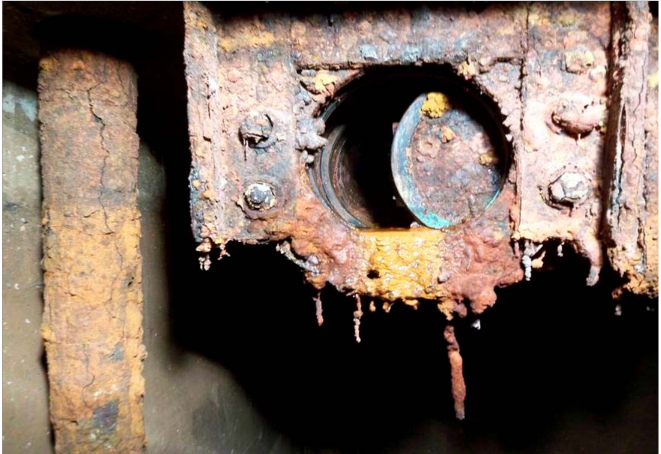
This April 2006 photo made available by the Nuclear Regulatory Commission in response to a public records request by The Associated Press shows a badly rusted valve in a containment that was initially a focus of concern as workers tried to find the source of leaks at the closed Indian Point 1 reactor in New York state. The leakage was eventually traced to spent fuel pools. been shut down since 1974. (AP Photo/Nuclear Regulatory Commission)
