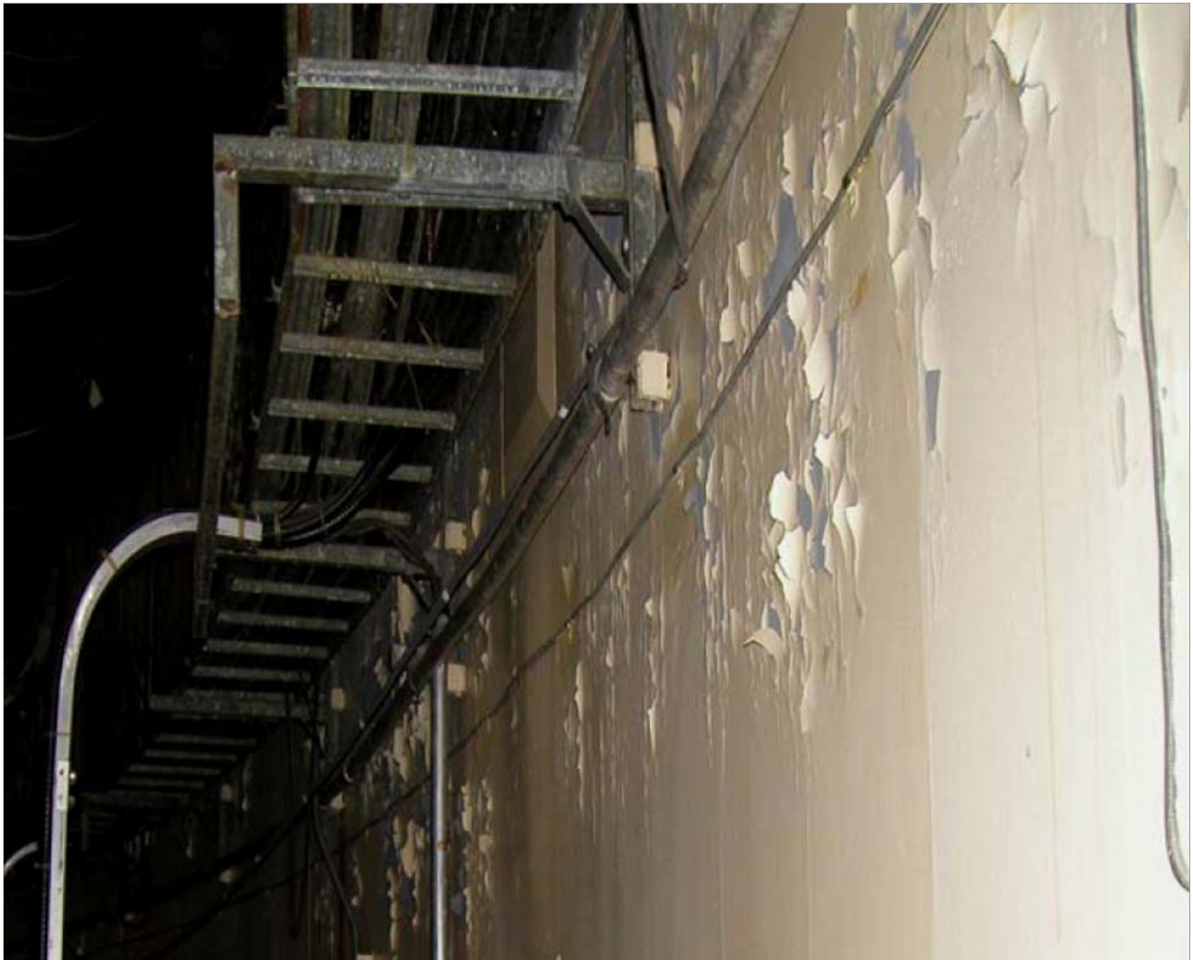
This spring 2004 photo made available by the Nuclear Regulatory Commission shows the finish peeling off a wall at the Oconee nuclear plant in South Carolina. An NRC inspector general's report in September 2007 said the operator had failed to manage this aging problem as it promised during relicensing. Even mundane deterioration at a reactor can carry harsh consequences. For example, peeling paint and debris can be swept toward pumps that circulate cooling water in a reactor accident. (AP Photo/Nuclear Regulatory Commission)
